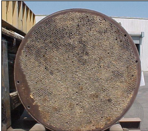
Clogged Tubesheet by Sever fouling
