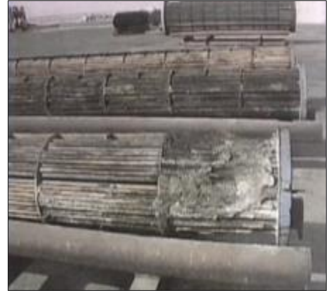
Coke fouling accumulation
